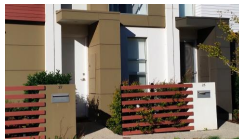
Meter box recessed & painted to match the wall minimizing visual impact.
