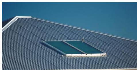
Solar hot water units must have on-ground storage tanks.
