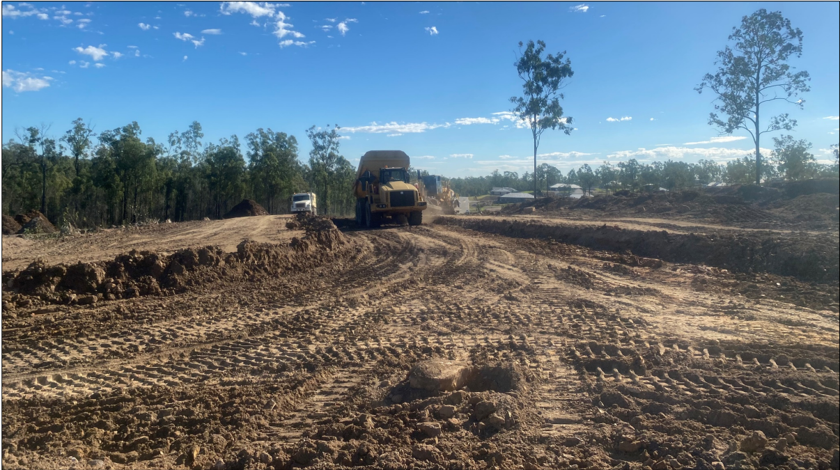
Figure 3 – Dump truck and compactor, to place, spread and compact fill material. (Taken 19/08/2020)
