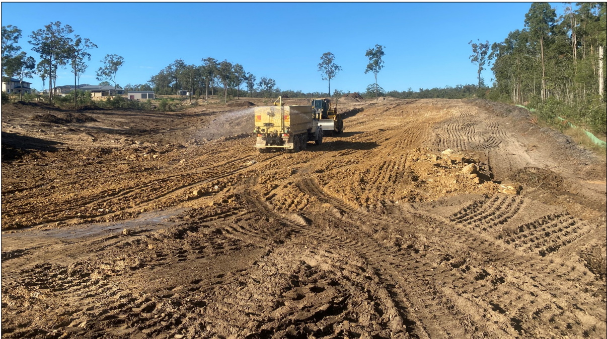
Figure 2 – Water truck and compactor. To moisture condition and compact fill material. (Taken 13/08/2020)
