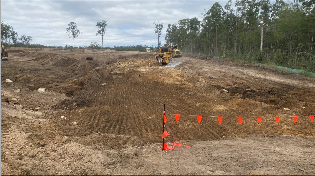
Figure 1 – Dump truck, dozer and compactor, to place, spread and compact fill material. (Taken 12/08/2020)
